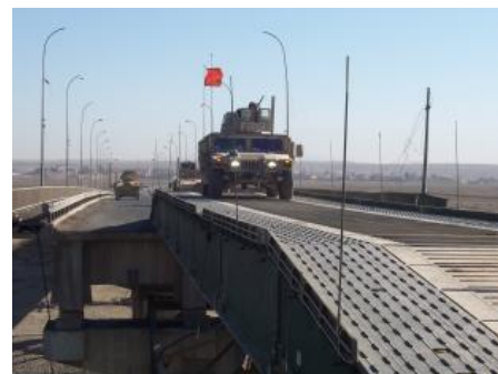
The Qayyarah Bridge on the Tigris River lost more than 100 feet of its span due to a truck bombing on Nov. 23, 2007.
